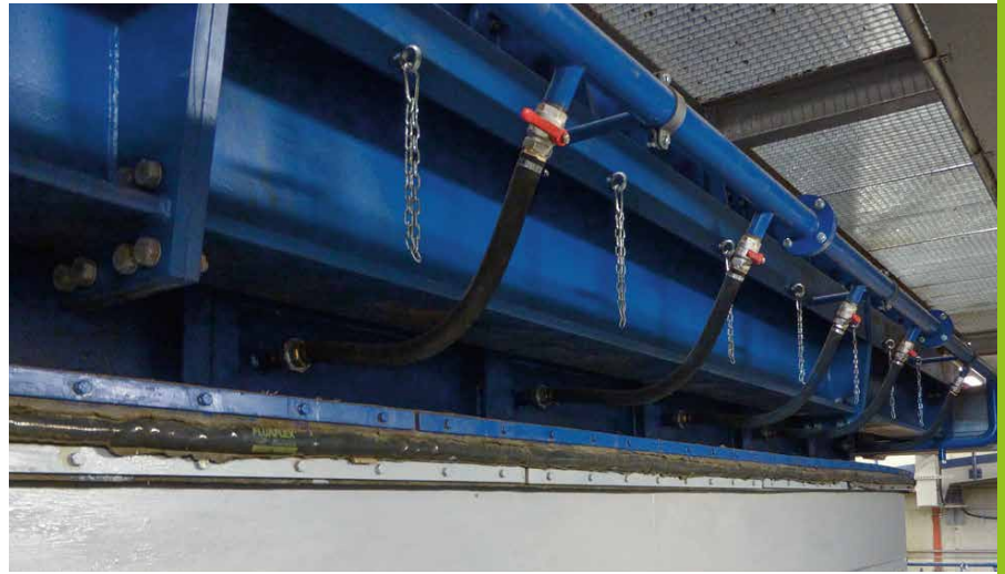
EfW plant Zistersdorf – water fed in from below
