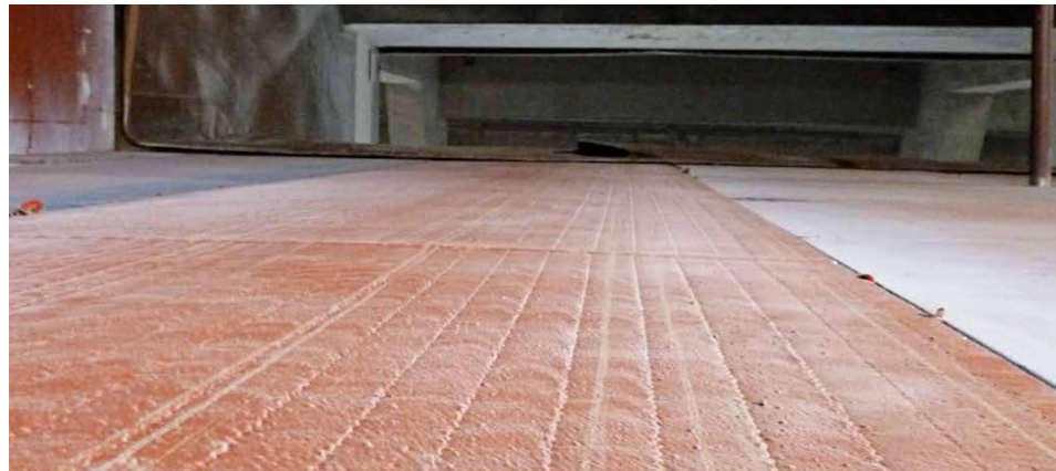
EfW plant Zorbau L2 – various materials were used for the inner surfaces of the bunker (cladding with alloy 12+4 and S235JR 16mm).
