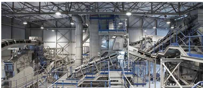
Dry mechanical bottom ash treatment (Poznan, Poland)
