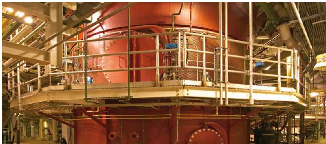
Metropolitan Council Environmental Services' Inova Fluid Bed St. Paul, MN, USA.
